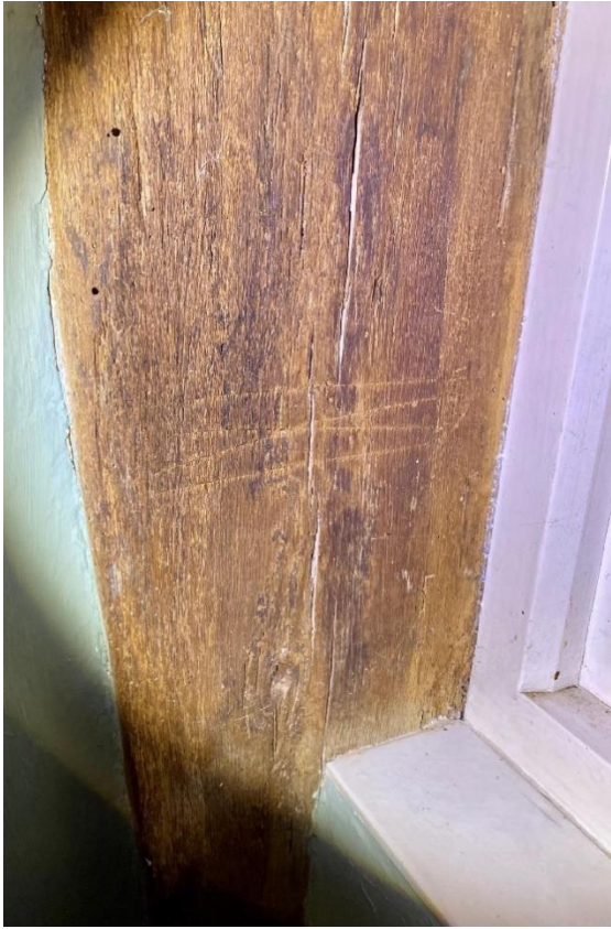
1 st floor south end of house (including bathroom) – 2 burn marks, one compressed butterfly by the window.
